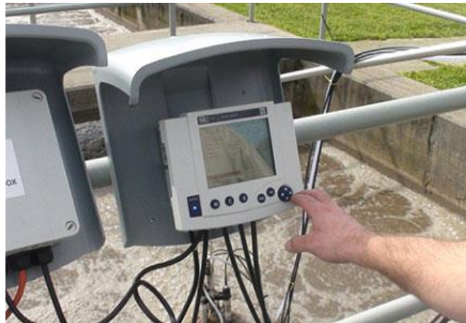
Figure 1 – Modern wastewater treatment plants produce plenty of data, but often are data graveyards.
